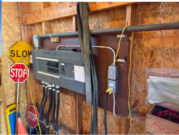
Main Service Panel
