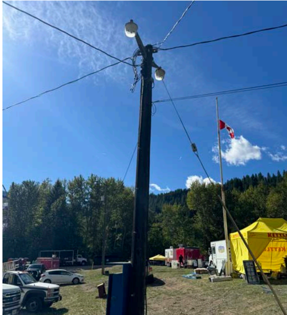
Distribution Pole Kitchen, Pavilion, Safety Shack, Event Distribution
