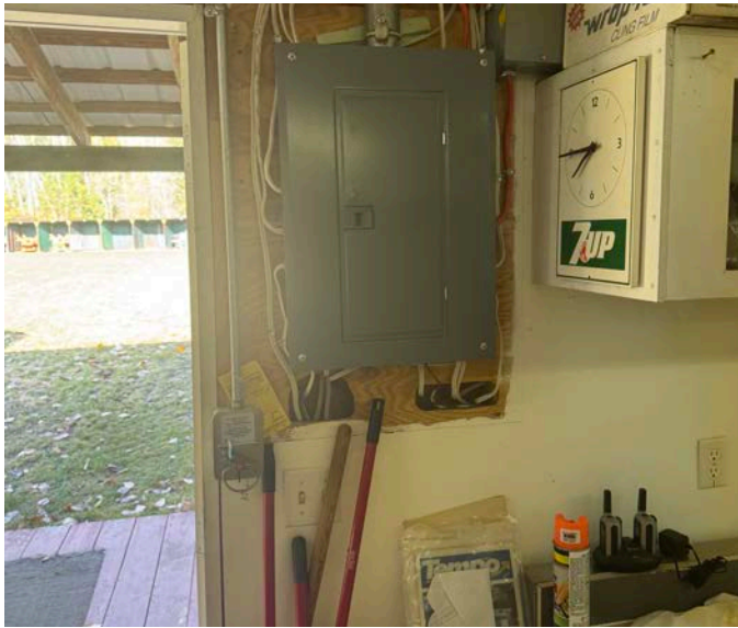
Kitchen Panel Exposed Wiring
