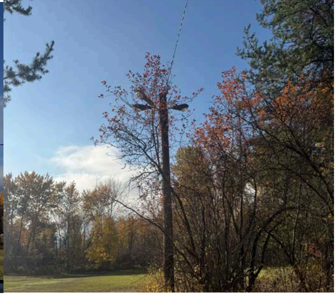
Parking Lot Lighting
