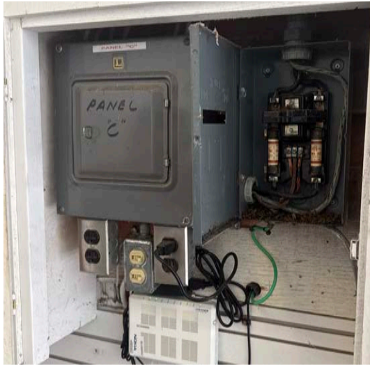
Pavilion Sub Service
