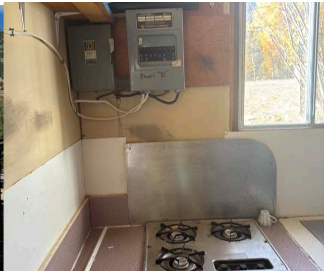
Safety Shack Panel and Wiring
