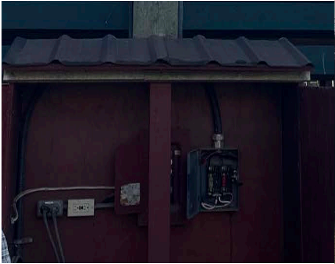
Box Stall Sub Panel
