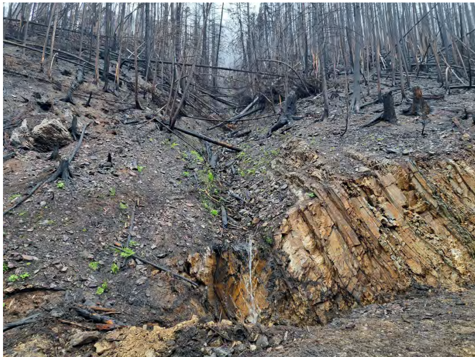
Photo 22: Shallow, steep gully susceptible to debris flows at Birnam FSR located within and downslope of a high burn severity area.
