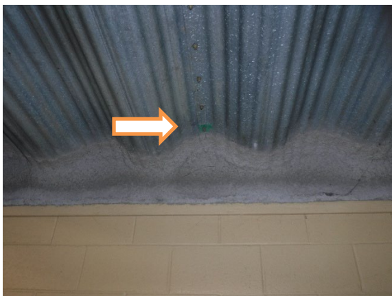
Sample C: Green sealant; south wall west on metal ceiling around last bolt adjacent to wall (500 ppm)
