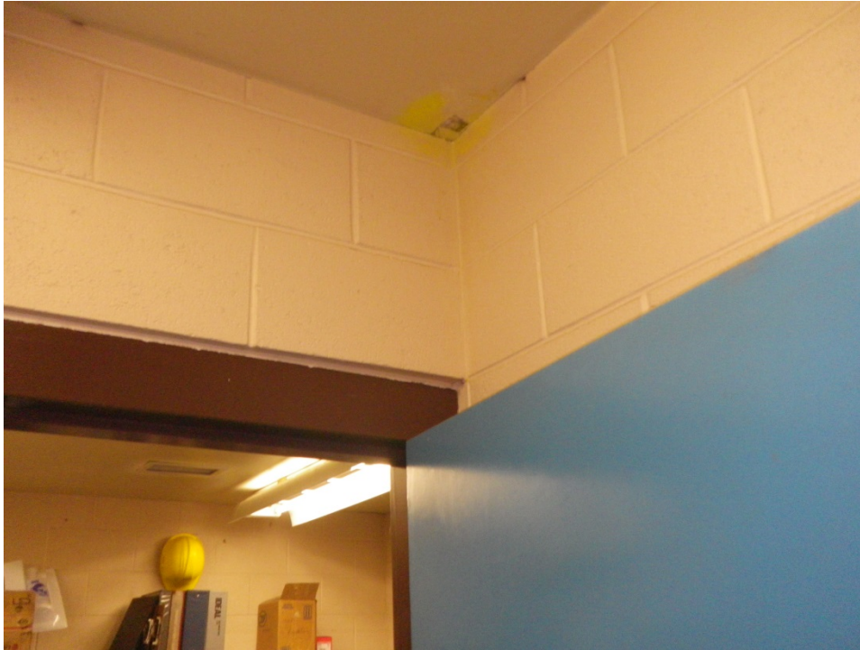
Sample 13: Maintenance foreman's office washroom; drywall mud sample on ceiling
