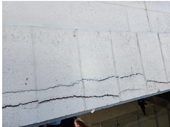
Figure 2: cracking visible on the header of door D69 – large swing door
