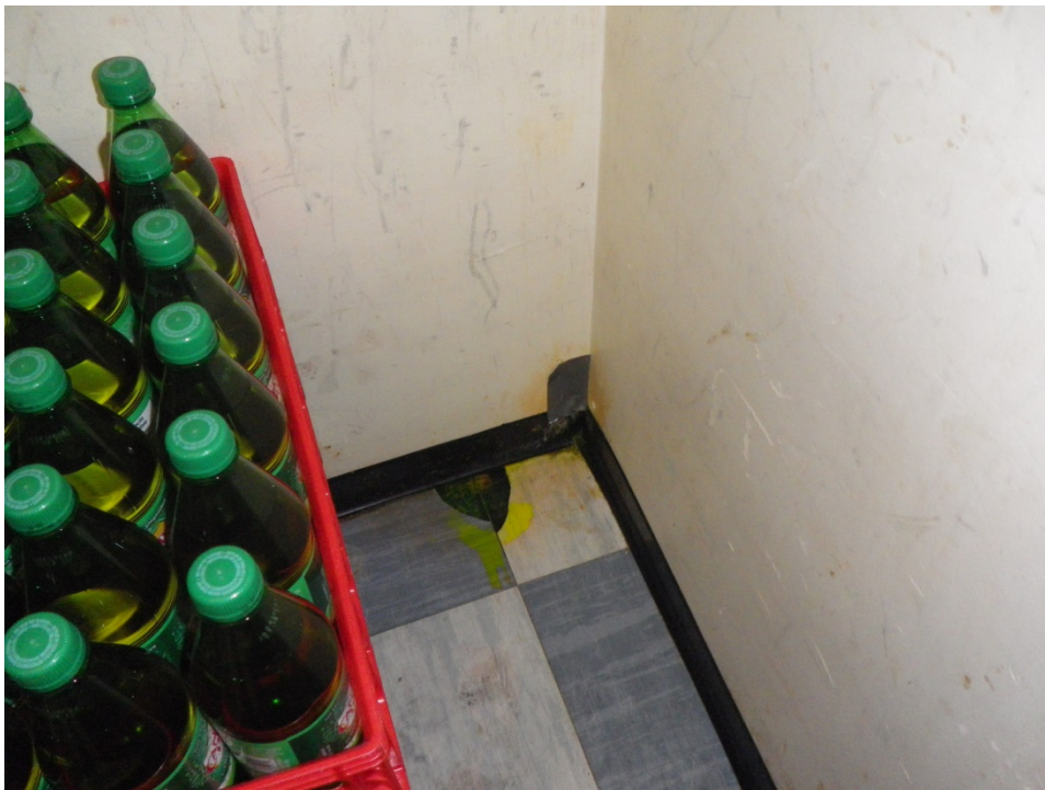
Sample 12: Drywall mud sample in kitchen dry good room
