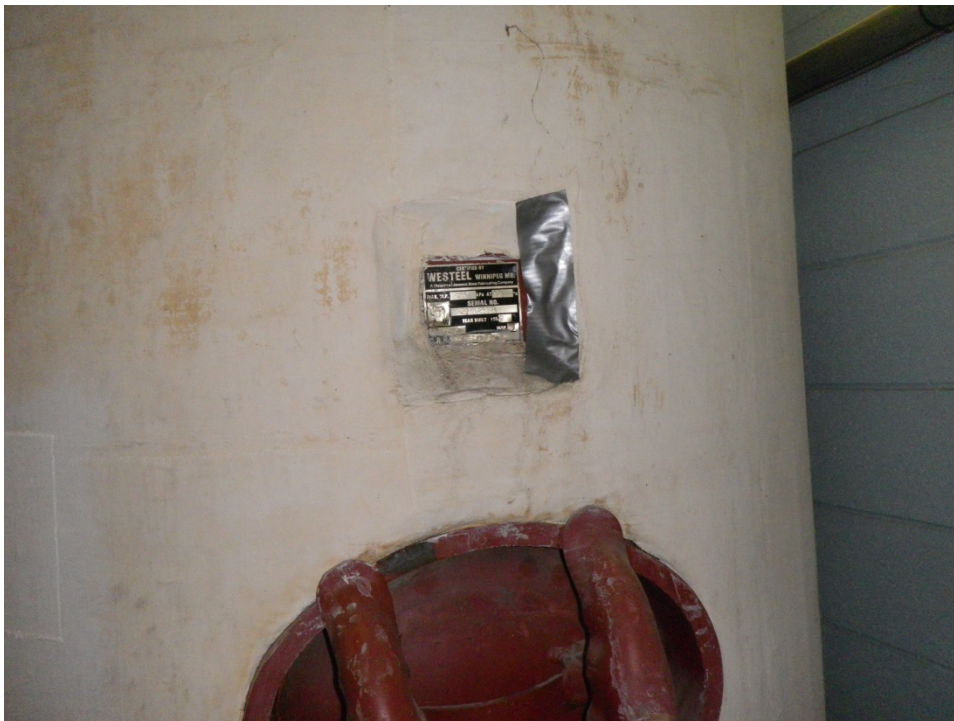
Sample 24: Pool mechanical room hot water tank; pipe wrap sample
