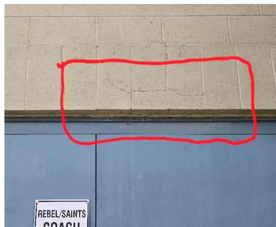
Figure 3: cracking visible on the header of door D72 – northern most door
