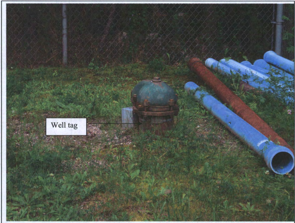
Groundwater well: RDCK Duhamel Water System May 19, 2006.
