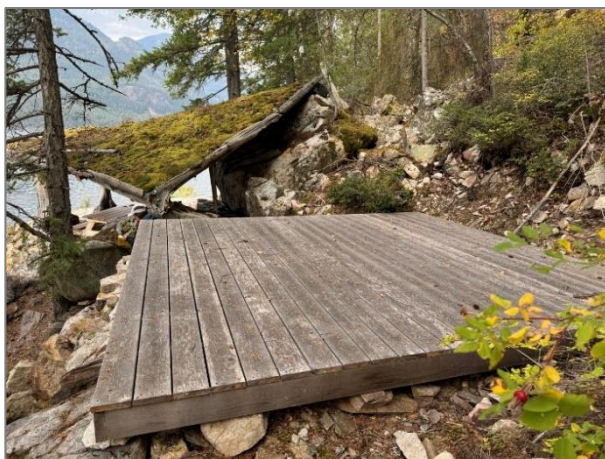
Photo 11. Existing tent pad with covered area in background. Note moss on roof. Oct. 15, 2024.
