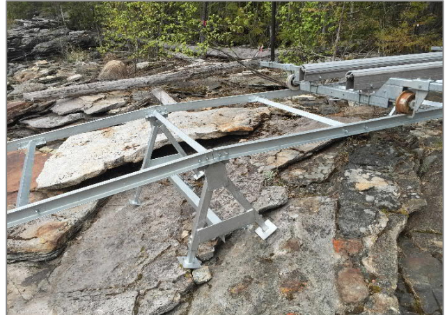
Photo 12. Example of marine rail support system.
