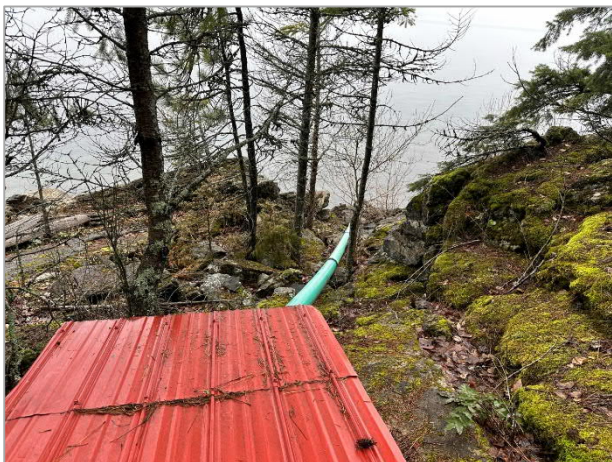
Photo 9. Existing water lines and pumphouse.
