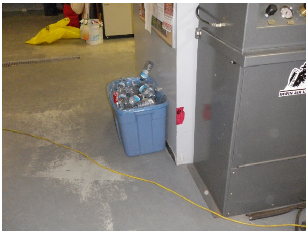
Figure 13: Sample 15, main floor, middle corner at tank fill, drywall joint compound
