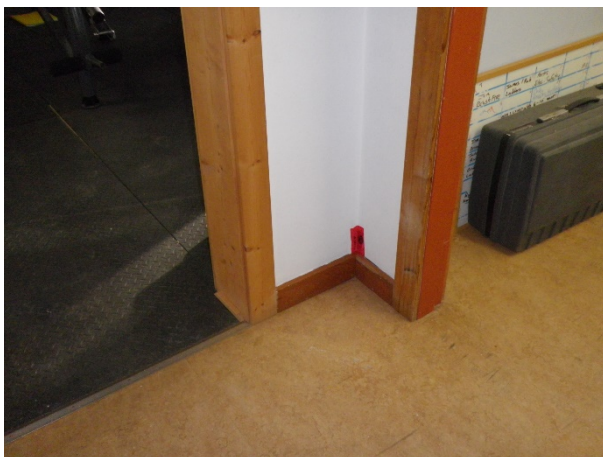
Figure 49: Sample 10, 2nd floor training room, SE corner, drywall joint compound
