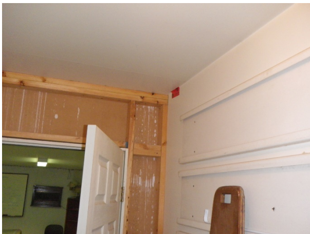
Figure 85: Sample 13, 2nd floor storage room, NW corner at ceiling drywall joint compound
