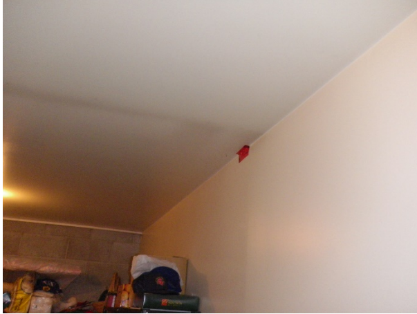
Figure 86: Sample 14, 2nd floor storage room, middle south wall at ceiling, drywall joint compound
