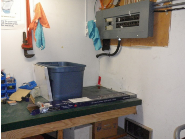
Figure 29: Sample 4, main floor SE storage room, drywall joint compound
