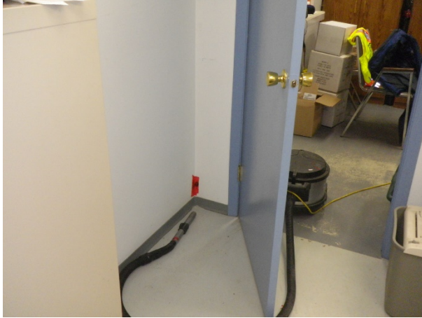
Figure 15: Sample 17, main floor computer room NW corner, drywall joint compound
