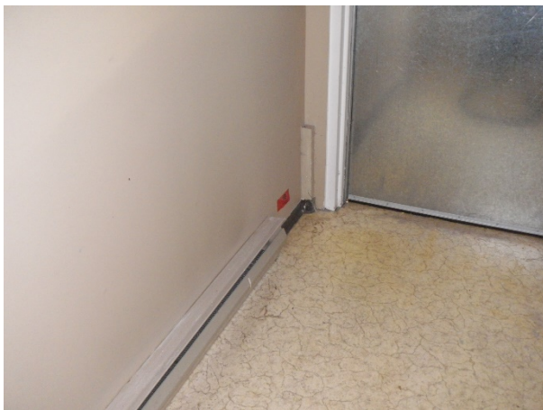
Figure 104: Sample F, main floor hallway by east exit, brown paint on wall
