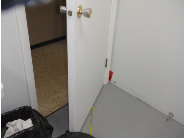
Figure 32: Sample 7, main floor men's washroom, NW corner, drywall joint compound
