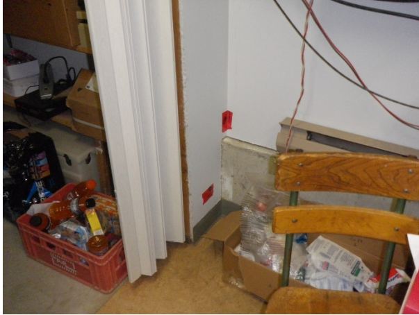
Figure 107: Sample A, main floor office, SW corner, light blue paint on wall
