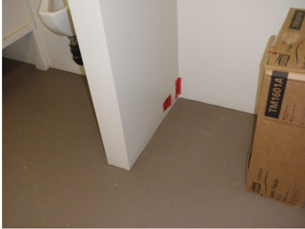
Figure 47: Sample 8, main floor, men's washroom south wall, drywall joint compound
