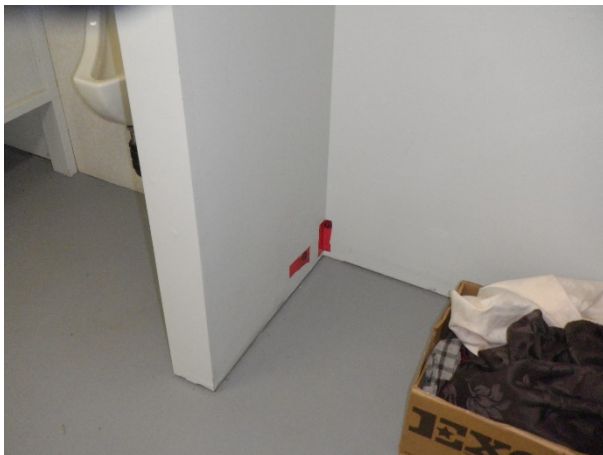
Figure 103: Sample E, main floor men's washroom, south wall light blue paint on wall
