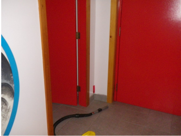
Figure 62: Sample 7, main floor hallway NW corner, drywall joint compound
