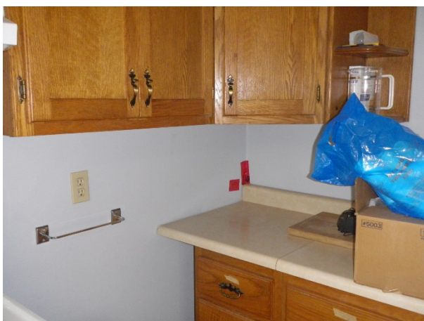
Figure 52: Sample 13, 2nd floor kitchen, SW corner, drywall joint compound
