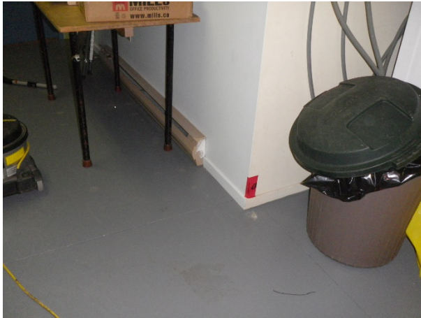
Figure 119: Sample A, main floor workshop middle corner, grey paint on concrete floor
