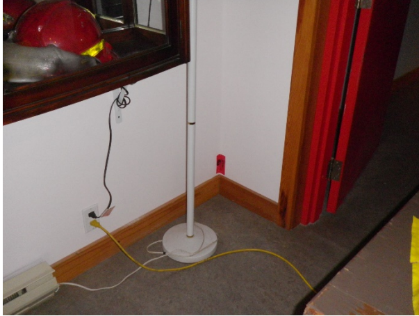
Figure 65: Sample 10, 2nd floor, recreation room, NE corner drywall joint compound
