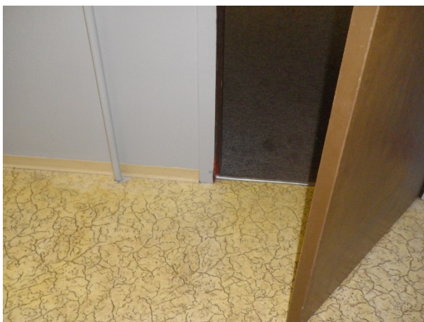
Figure 98: Sample F, 2nd floor kitchen, north door trim, brown paint on metal trim (805ppm)
