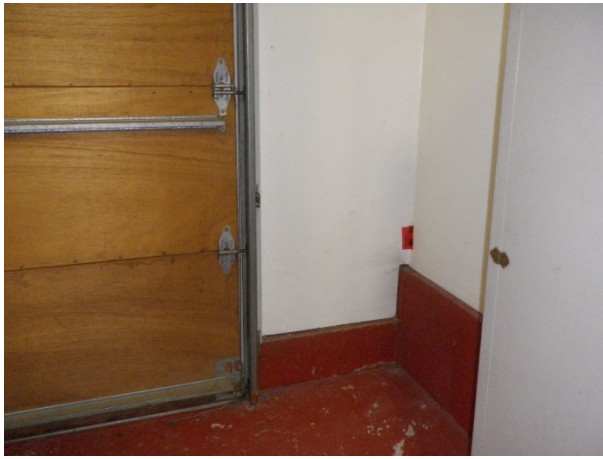
Figure 16: Sample 1, main floor main bay, SE corner, drywall joint compound
