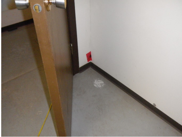
Figure 96: Sample D, main floor men's washroom, NE corner floor, grey floor paint on concrete (2510 ppm)
