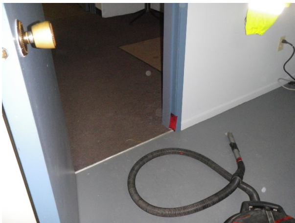
Figure 121: Sample C, main floor office door trim, dark blue paint on wood door trim
