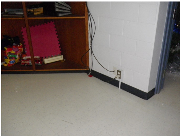
Figure 81: Sample 9, 2nd floor family room, NW corner vinyl floor tile
