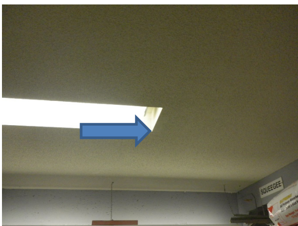
Figure 14: Sample 16, main floor, wet side ceiling at west light fixture, texture coat
