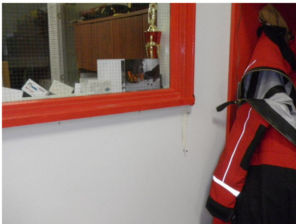
Figure 101: Sample C, main floor main bay, SW corner, red paint on window trim (9280 ppm)
