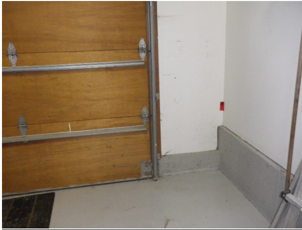
Figure 26: Sample 1; main bay NE corner, drywall joint compound
