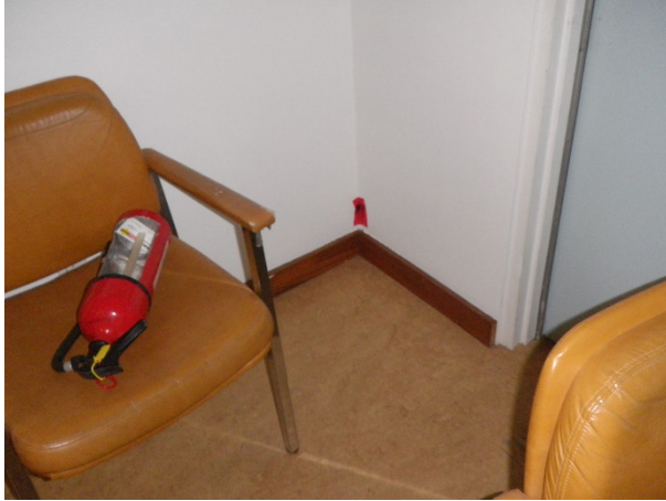
Figure 50: Sample 11, 2nd floor training room, SE corner, drywall joint compound
