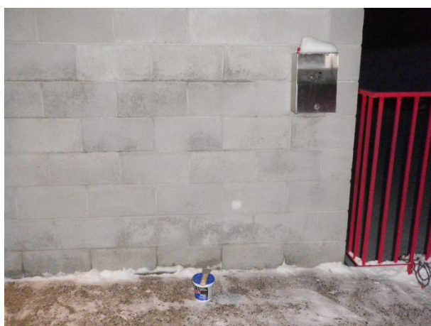
Figure 70: Sample 15, 2nd floor, patio off recreation room, exterior cinder block wall vermiculite insulation (trace actinolite asbestos)
